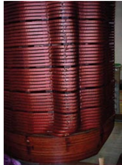
Winding defects shown in coil displacement
