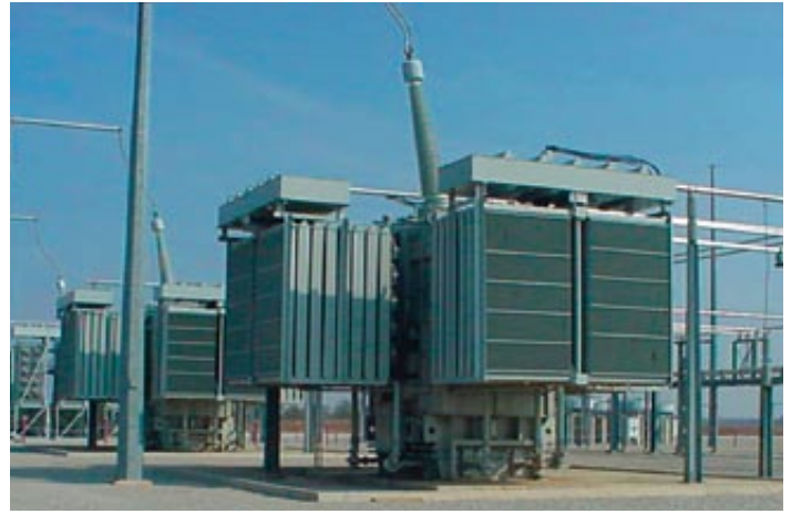
ABB can diagnose your power transformers and provide you with the information you need to make effective O&M decisions
